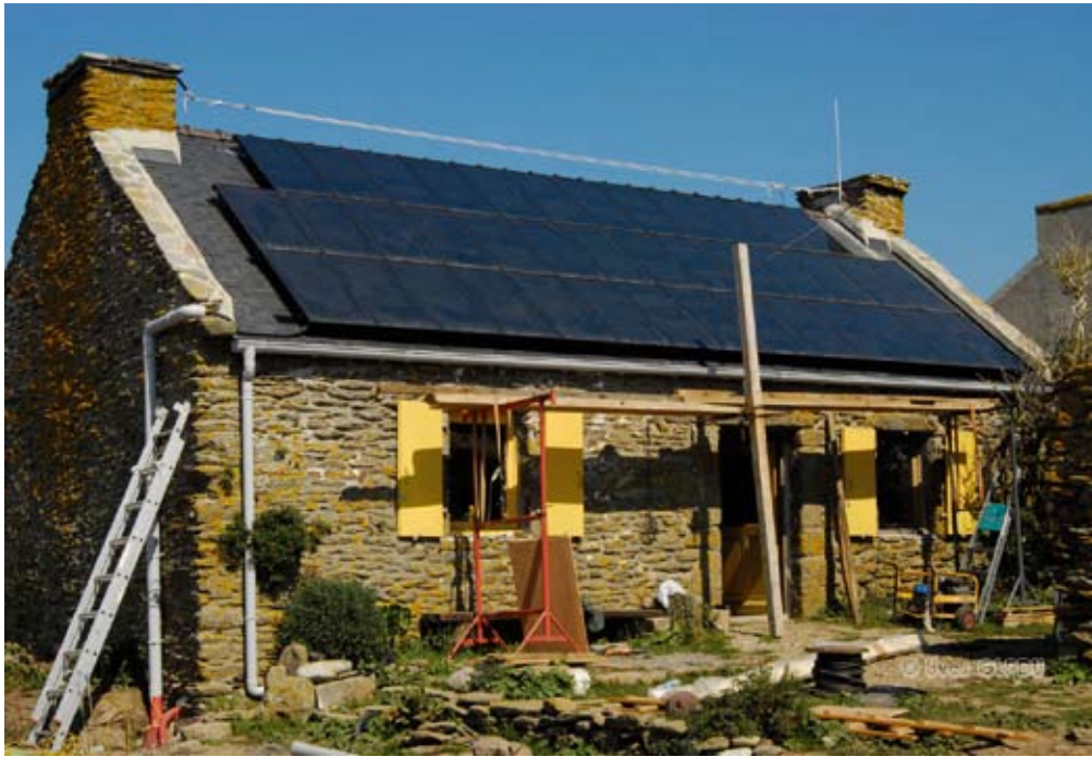
Iroise Archipelago, Ty-Kozh, Solar panelling
